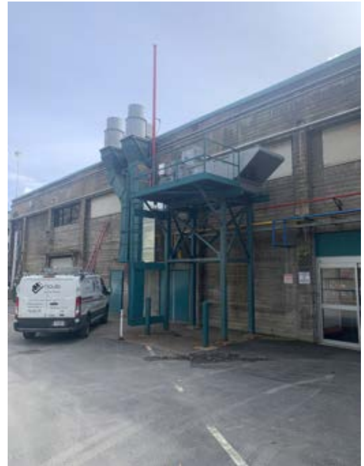
TMC – Plant HVAC Unit
