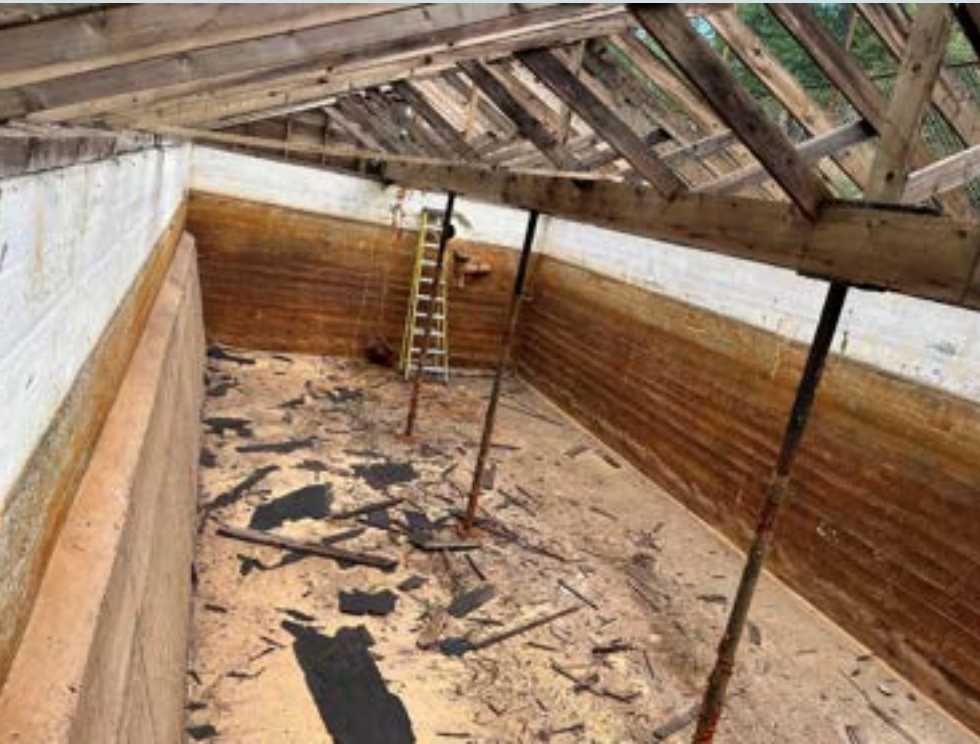
Lookout reservoir – Old roof
